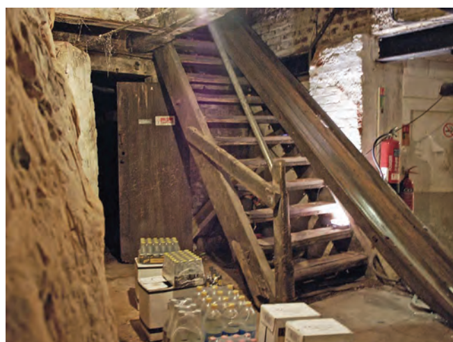
The entrance to the suspected air-raid shelter is squeezed between a bulging sandstone wall and a barrel ramp and staircase
